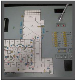
Control Panel for Jail in Jail Control
